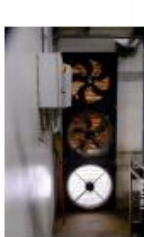
Figure 3. Forced ventilation fans
