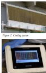
Figure 4. Air quality and ventilation parameter control panel
