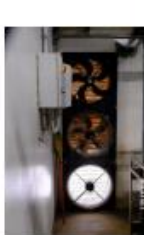
Figure 3. Forced ventilation fans
