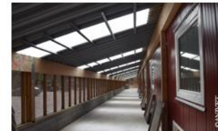
Veranda with fabric netting with small mesh size at sides and roof tiles alternating in transparency.
